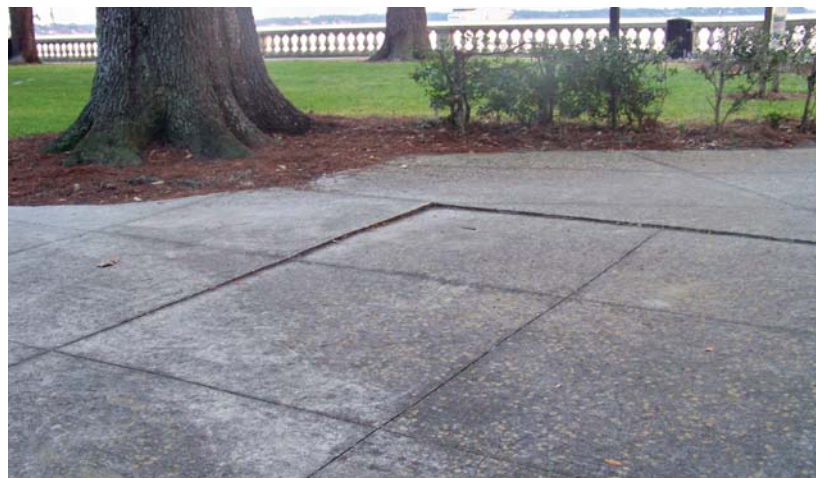
Walkway starting to lift, despite presence of cutout.
