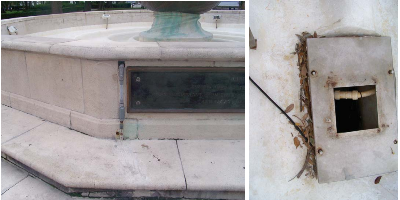
Old electrical work mars some of the fountain's cast stone cladding (left); the current pump vault is undersized and the pump out of commission (right). Fountain restoration must address plumbing systems, controls, the basin lining and full restoration / repair of all of the cast stone work.
