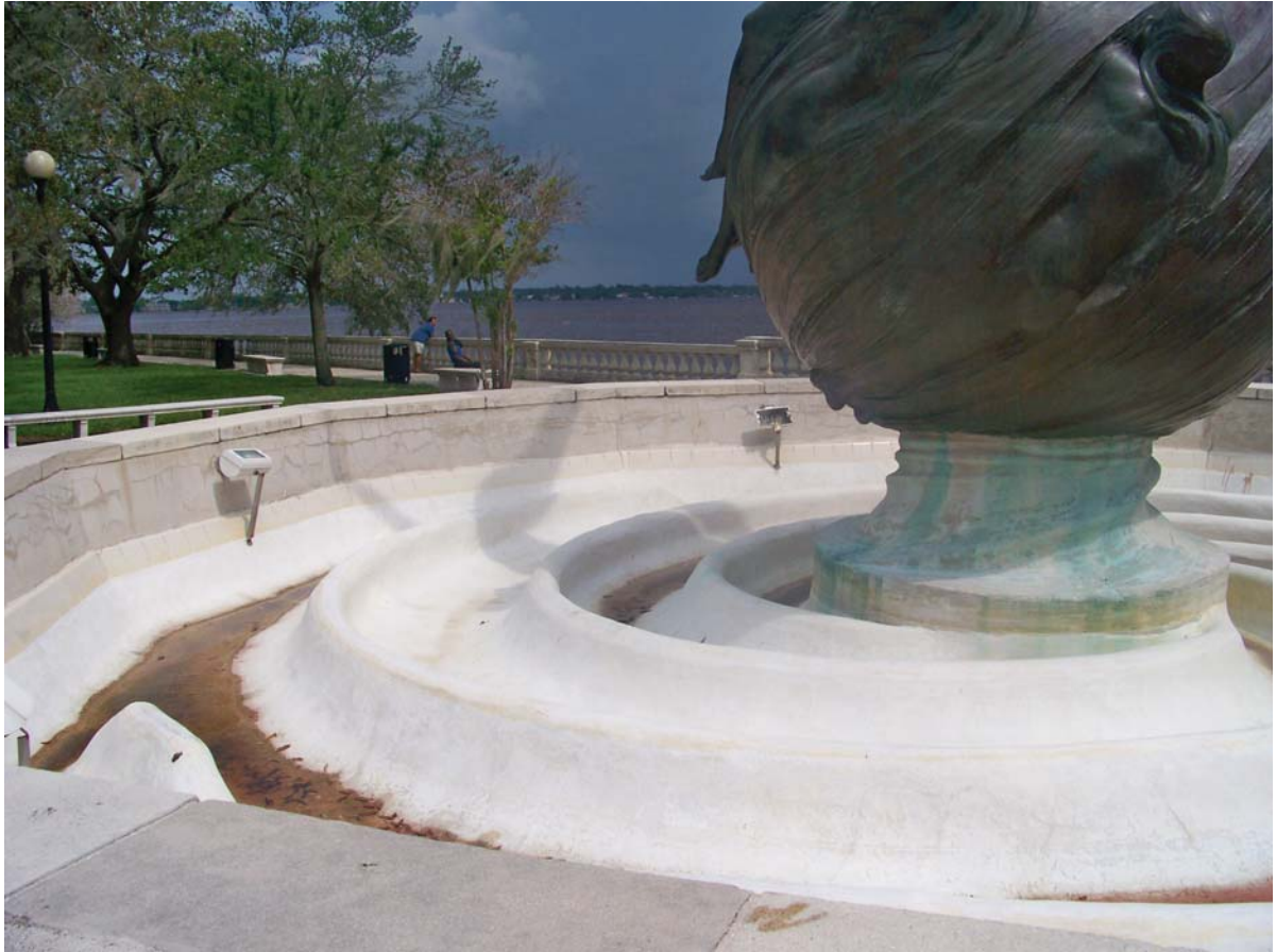
The installation of lights and electrical conduit in the fountain basin wall has damaged the interior surface and is visually intrusive.
